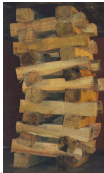
this wooden crib is providing approximately 100 tons of support and has allowed about 16" of convergence.
