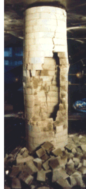
At 1.80" of convergence the support value is lost. In other areas of a mine, maintaining a seam height is not as important and wooden cribs may provide all the support needed. With more floor to roof convergence.
